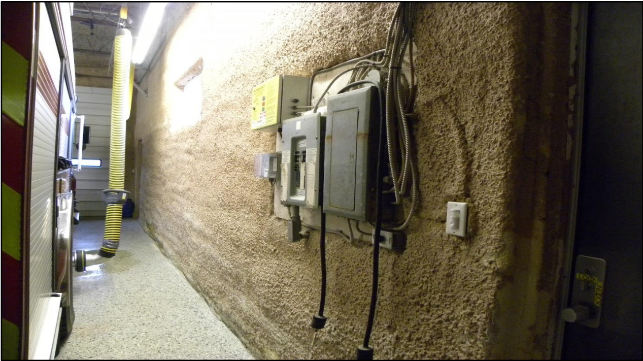
Apparatus parked close to the overhead doors
