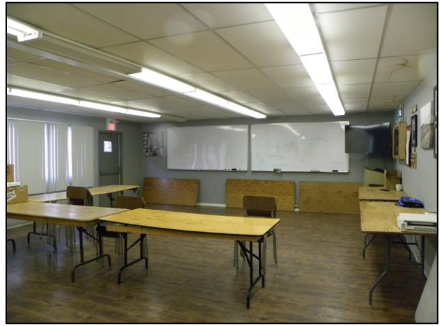
Water stains on ceiling tiles
